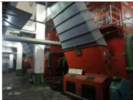
3台20t/h燃煤蒸汽锅炉
